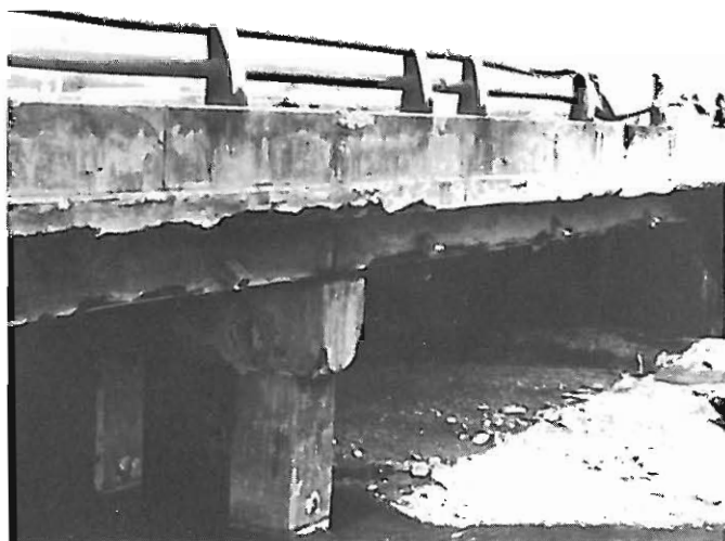
Mill Creek Bridge on Highway 71 in Fort Smith following fire.
