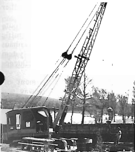
Construction crews assemble one of the two barges used in the ferry operation at Edgemont.
