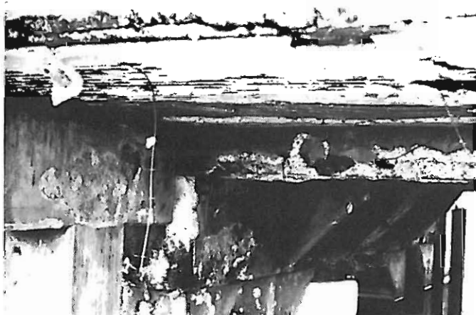
Close-up view of damage caused by fire to the Mill Creek Bridge on Highway 71 in Fort Smith.
